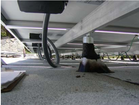
Figure 5 (incorrect) Flex exposed to physical damage
