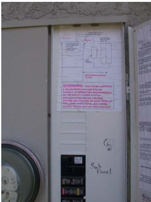
Figure 13 Sign at service entrance required by 702.8
