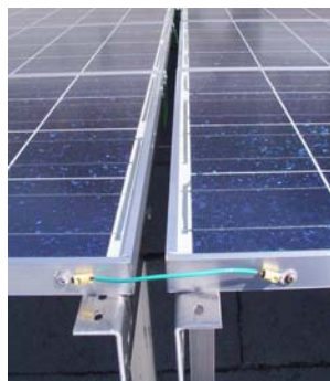
Figure 3 (incorrect) Need consistent path for ground
