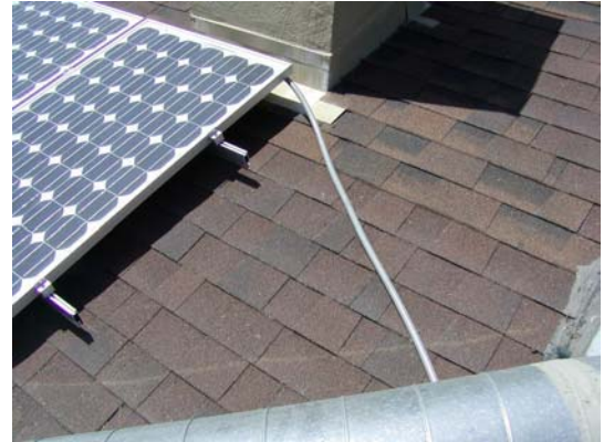
Figure 6 (incorrect) Flex conduit run without support
