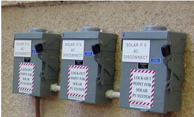
Figure 12 PV System Disconnect Signs
