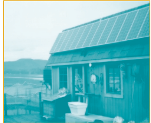
▲ This PV-powered aquaculture facility is on an island off Canada's west coast.
