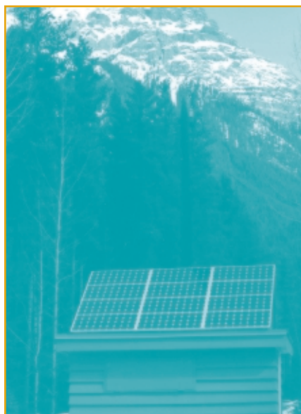
▲ The autonomous PV system in Yoho National Park, British Columbia, supplies electricity for the amphitheatre projector and recharges the batteries of a golf cart that the staff uses to collect camping fees. Photo courtesy of Sovran Energy Inc.
