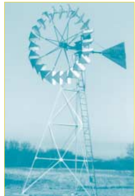
▲ Mechanical water pumping system.
